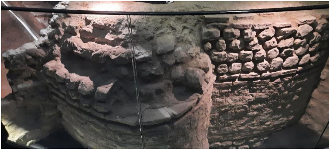
Figure 9: © View of sandy limestone (Kentish ragstone) used as foundations of the Temple.
